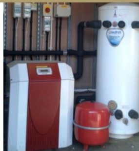
Ground source heat pump, Cardiff nursery school ©BGS
